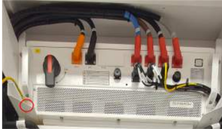
Figure 5-24 Position of Grounding Cable
