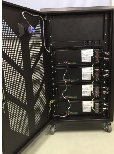
Communication cable connection
